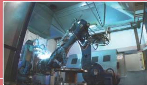
All welding of the frame and components is done entirely robotically in robotic chambers.
